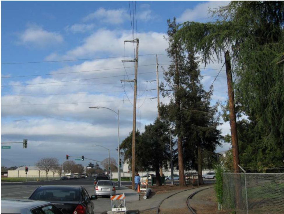
Those 115 KV Power lines (note our iron pole on the ground)
