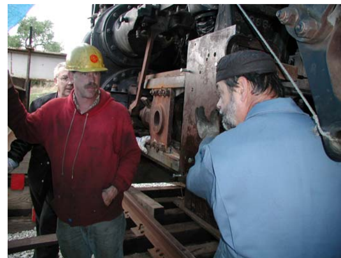
Tom Anderson and John Ezovski setting up a steel plate to mount the magnetic base drill
